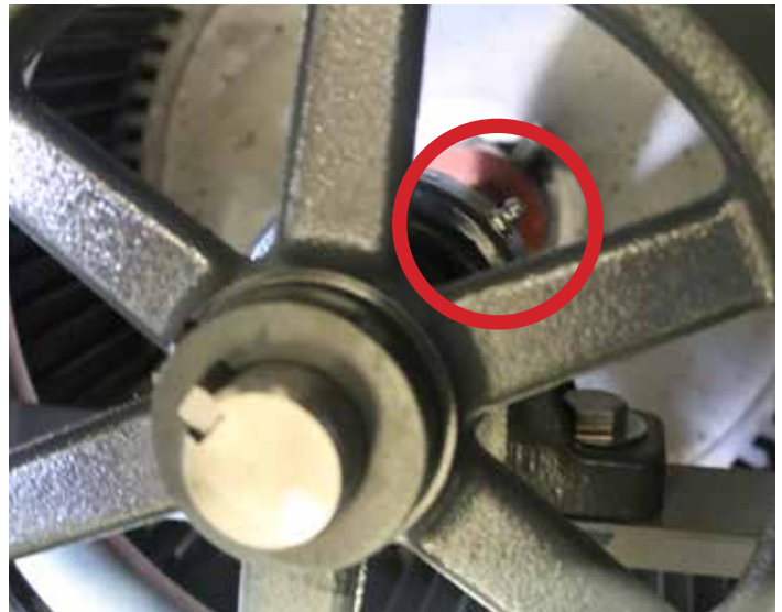
Figure 6 – Evaporator Blower Lubrication
